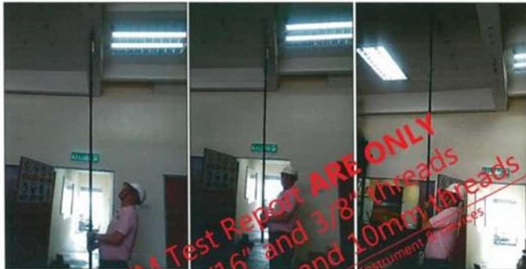
Photo A.2.1 : Installing Fastener Shooting Nail to ceiling beam and ceiling slab.
