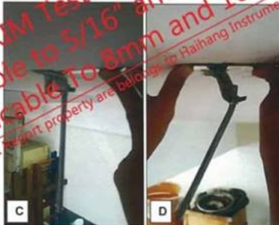
Photo A.3.2 : Filler gauge unable to pass through at 1.55mm for (C) and 0.50mm for (D).
