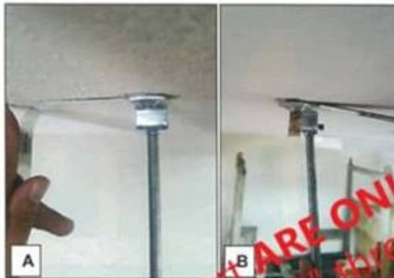
Photo A.3.1 : Filler gauge unable to pass through at 0.05mm for both (A) and for (B).
