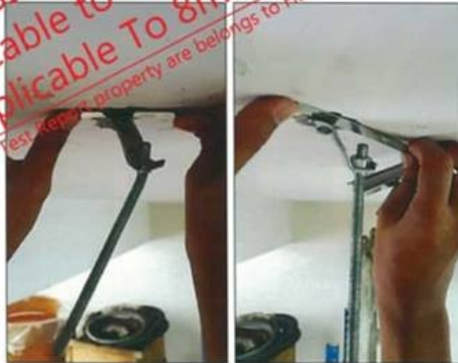
Photo A.7.3 : Gap measured after pull out for sample (C) and (D) at ceiling slab.
