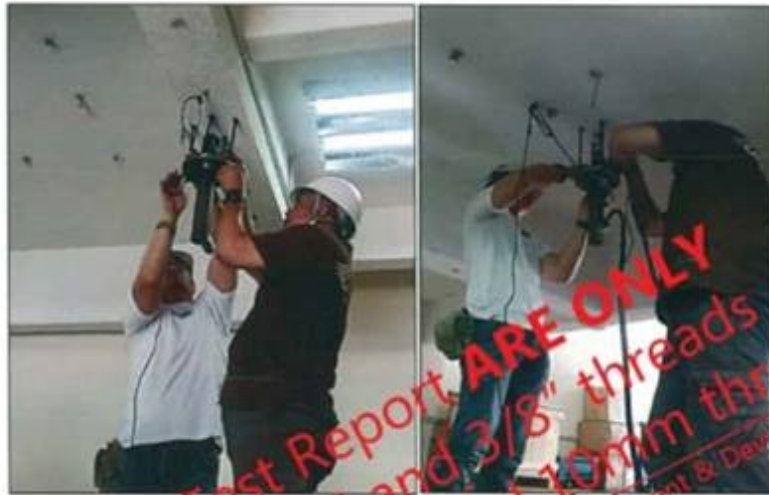
Photo A.4 : Installing tester unit and appropriate pull out adaptor at ceiling beam and ceiling slab.
