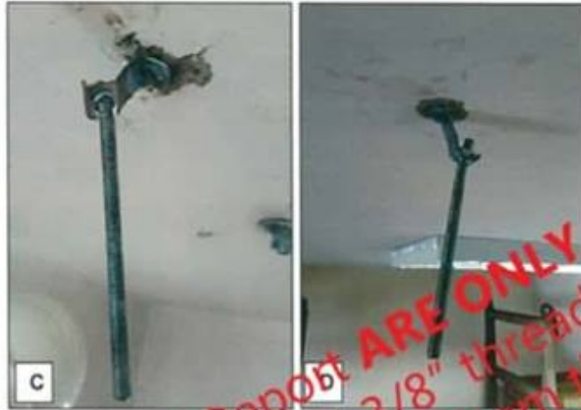
Photo A.7.2 : Fastener Shooting Nail after pull out for samples (C) and (D) at ceiling slab.
